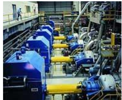
4 pulp refiners each with 6.5 MW motor
